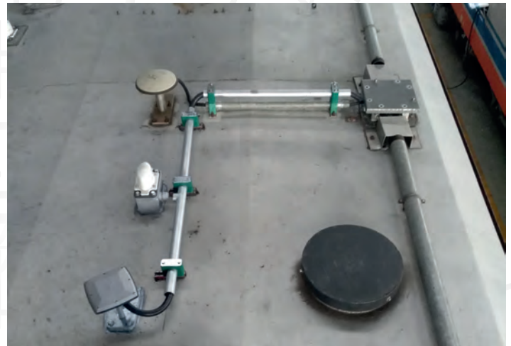
Antennas to receive DGNSS/RTK correction
